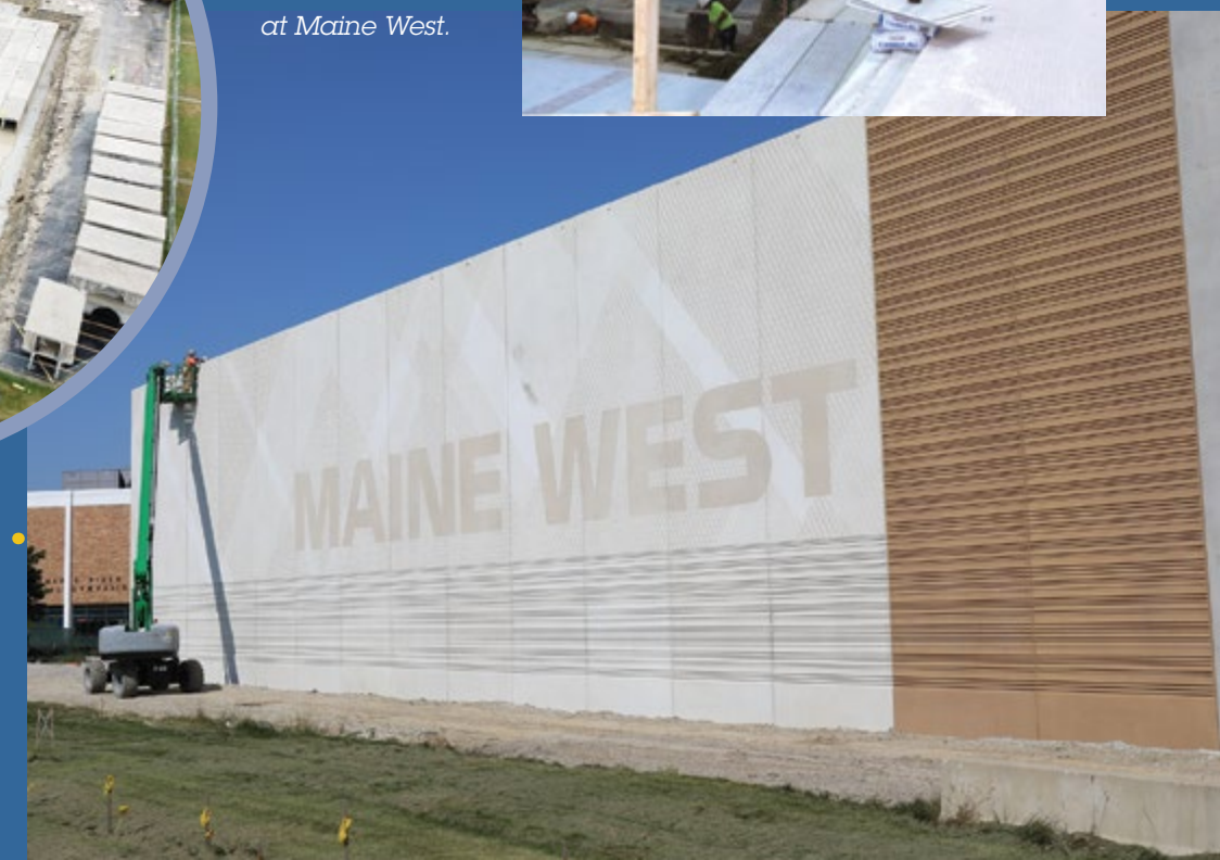
A view of the outside of the new Maine West field house as it begins to take shape.
