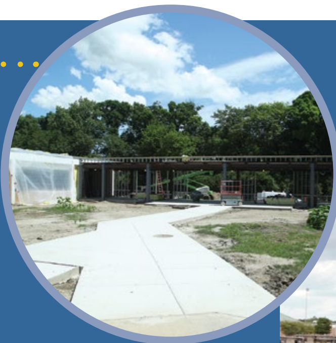
The construction of a new hallway that will connect the main building at Maine South with A wing is in progress.
