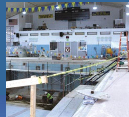
The swimming pool renovation at Maine West will deepen the pool and replace the original pool gutter system.
