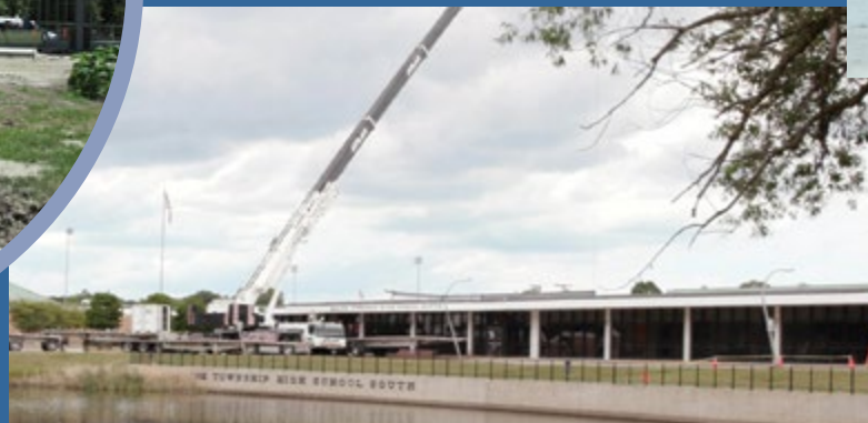
A crane delivers materials to the former courtyard as that space is converted into a new cafeteria at Maine South.
