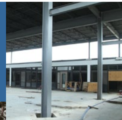
With steel supports installed, work begins on transforming the former courtyard into space for the new cafeteria at Maine South.
