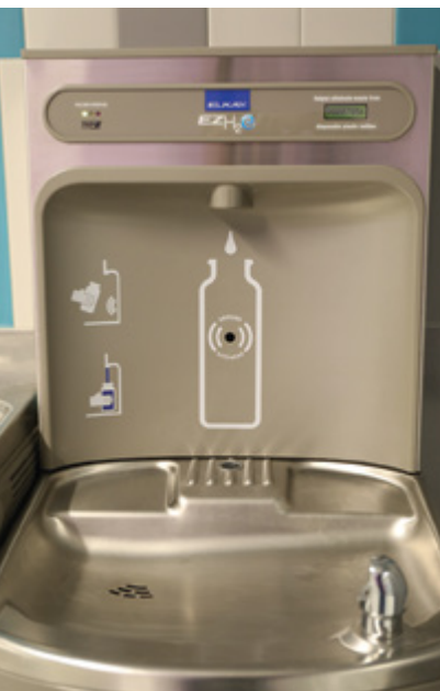
The new water fountains all include the ability for students and staff to refill their water bottles to reduce the use of plastic bottles.
